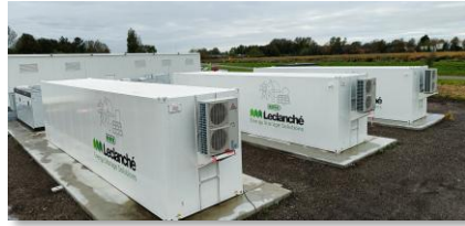
S4 Energy Noord Holland, Netherlands Frequency regulation System energy: 9 MWh
