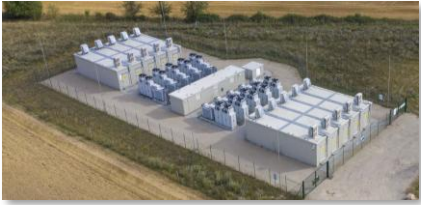
Enel Green Power Cremzow, Germany Frequency regulation System energy: 34 MWh
