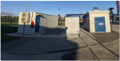
Veolia Gas Power Plant Levice, Slovakia Secondary Frequency Control System energy: 5.2 MW / 2.9 MWh
